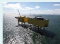
Commissioning two HVDC platforms for Siemens Energy in the German North Sea
