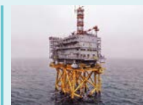
HKZ Alpha and Seagreen topside HVAC units installed
